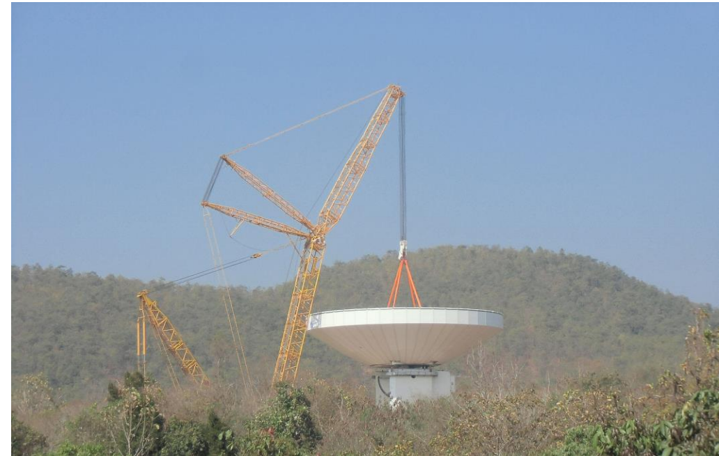
The 250-tonne reflector was placed on the steel substructure during the big lift
